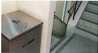
Waste collection bins on staircase landings
